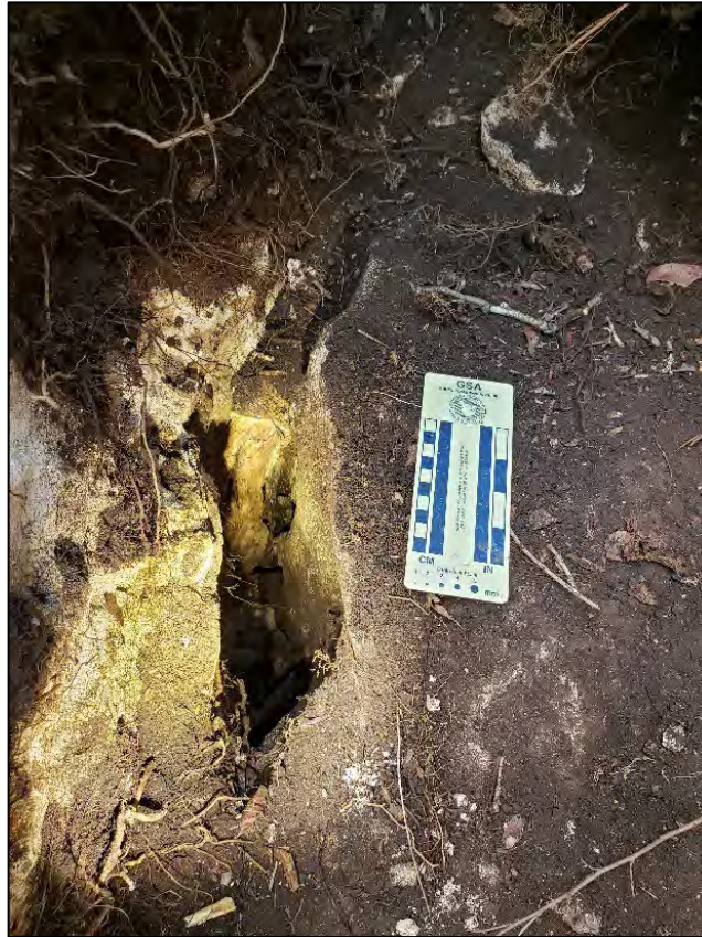
Figure 22. Floor drain following a fracture exposed after excavation.
