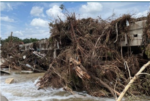
Big Sandy Bridge - debris buildup
