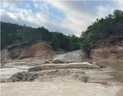
Cow Creek Road - low water crossing washed away
